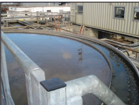
In this thickener, polymer is combined with the slurry prior to dewatering, stockpiling and removal of the dredged material.
