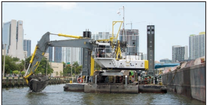
Bean's multi-purpose dredge Barredor Del Rio in backhoe mode in the Miami River. It will fill the barge in the right of the photo, which will be conveyed to the material processing site. The symbolic "last scoop" of the project was taken on October 15, 2008. The five year, 88 million dollar contract removed 750,000 cubic yards of contaminated sediments from a 5.5-mile stretch of river.
