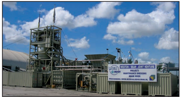
The entrance to the material treatment plant on the north shore of the Miami River. This is a portable plant and can be dismantled and moved to another project.
