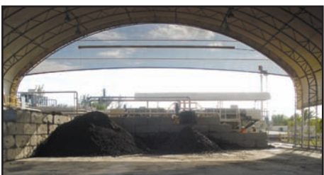
The stockpiled material is covered until hauled to a safe disposal site by truck.
